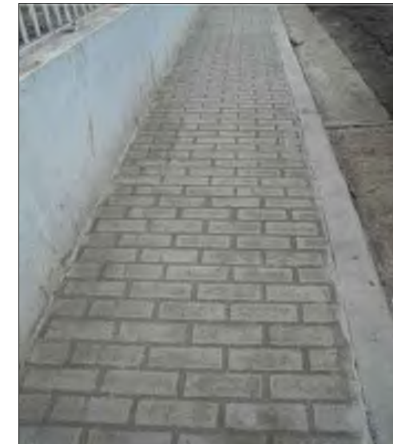
DECORATIVE CONCRETE STAMPED PATTERN: RUNNING BOND BRICK COLOR: 'DAVIS' INTEGRAL COLOR #860 'COBBLESTONE'
