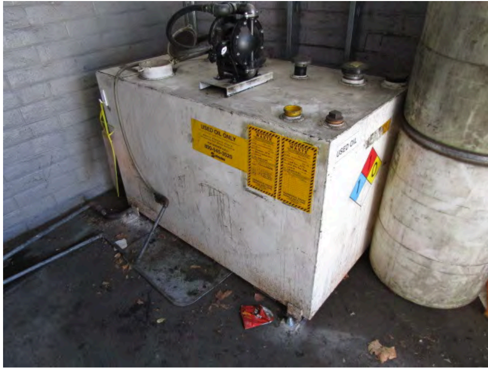
13. Waste oil AST in the enclosure on the southern side of the building
