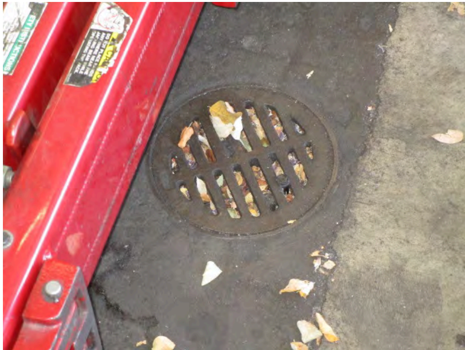
26. Floor drain in the automotive service area
