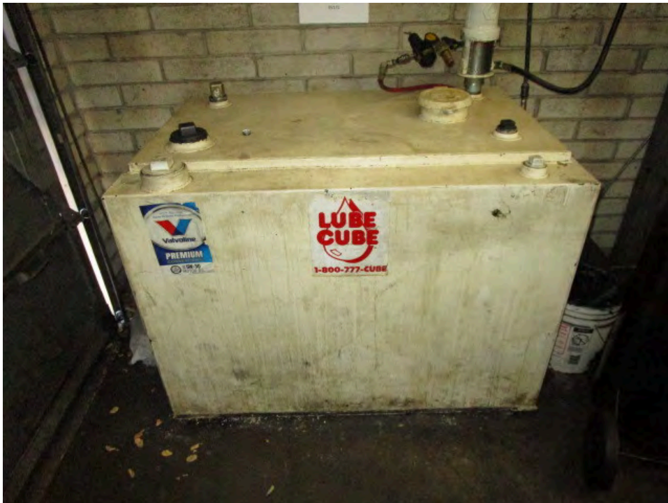
34. New oil AST in the store room
