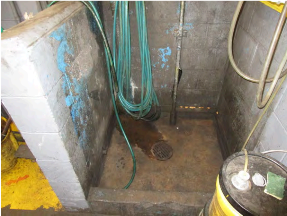
35. Floor sink in the automotive service area
