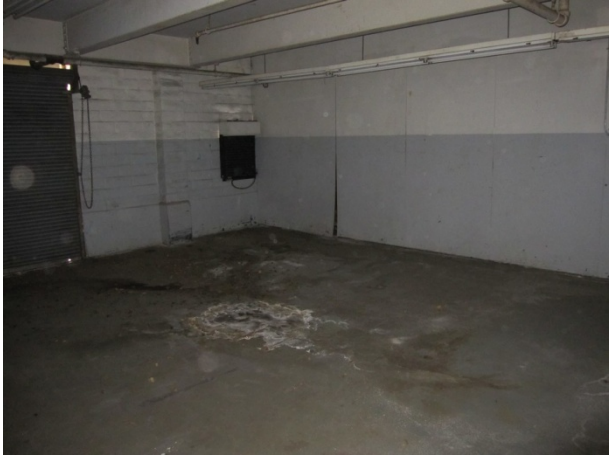
Photograph 17. Staining on floor of battery room at SAC.
