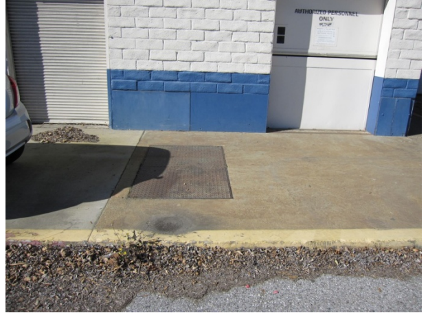
Photograph 24. Steel cover of acid neutralization chamber adjacent to battery room at SAC.
