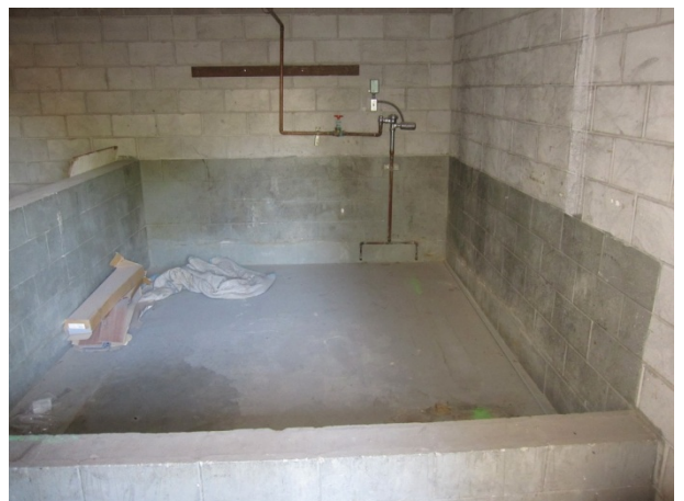
Photograph 28. Secondary containment area at JC Penney.
