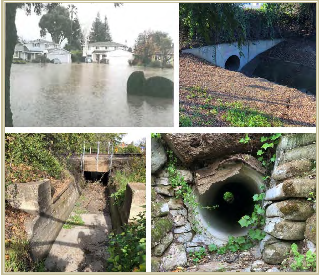
Figure 1-2: Elm Court Flooding and Storm Drain Structures in Cupertino
