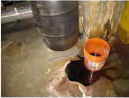
Photograph 11. Oily water on floor of mechanical room at Cupertino Ice Center.
