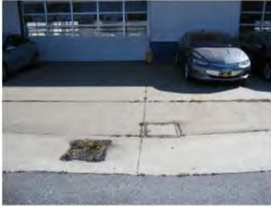
Photograph 23. Concrete access cover (near storm drain) at the suspected waste oil UST location at SAC.
