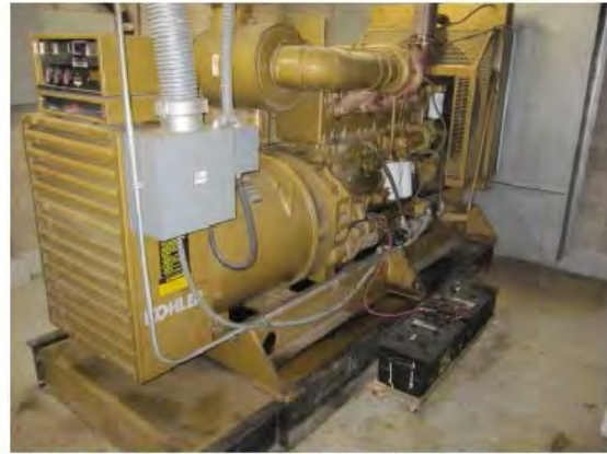
Photograph 6. One of three on-site emergency generators.
