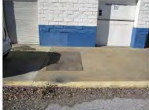
Photograph 24. Steel cover of acid neutralization chamber adjacent to battery room at SAC.
