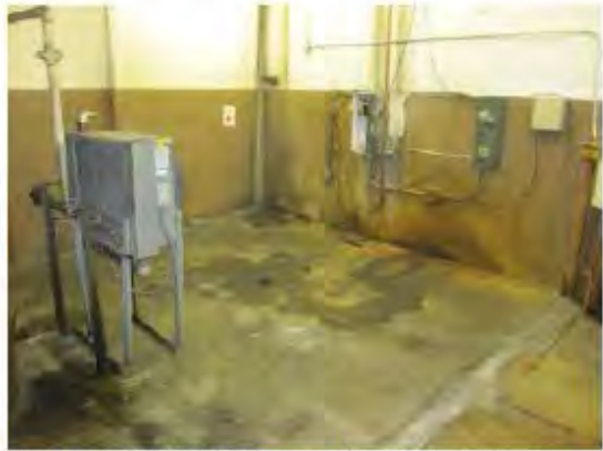
Photograph 20. Staining on floor near drain at former compressor location in basement at SAC.
