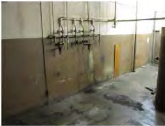
Photograph 19. Remnant distribution piping and staining on floor in basement at SAC.
