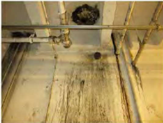
Photograph 21. Waste oil drain in floor slab, capped drain pipe in wall and wall staining in basement at SAC.
