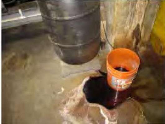
Photograph 11. Oily water on floor of mechanical room at Cupertino Ice Center.
