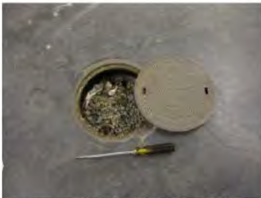
Photograph 27. Former hydraulic lift filled with pea gravel at JC Penney.
