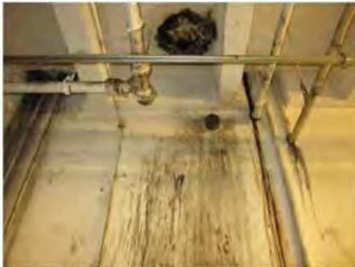
Photograph 21. Waste oil drain in floor slab, capped drain pipe in wall and wall staining in basement at SAC.
