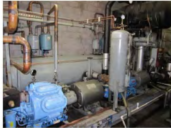
Photograph 8. Refrigeration equipment at Cupertino Ice Center.
