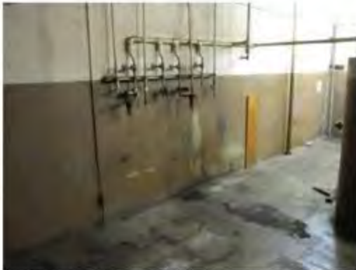
Photograph 19. Remnant distribution piping and staining on floor in basement at SAC.
