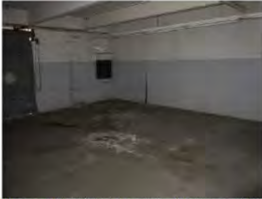
Photograph 17. Staining on floor of battery room at SAC.
