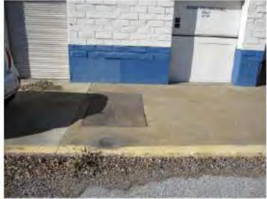
Photograph 24. Steel cover of acid neutralization chamber adjacent to battery room at SAC.
