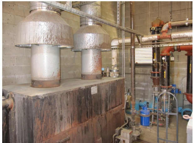
Photograph 12. Natural gas fueled boiler at community building.
