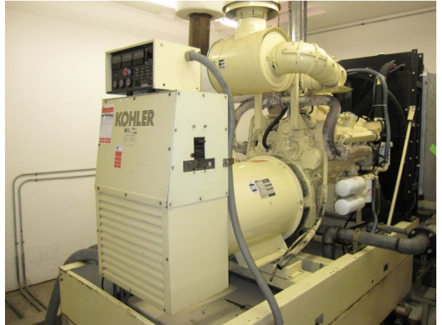
Photograph 4. Emergency generator at the health care center.
