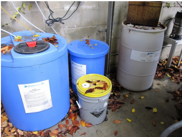
Photograph 11. Water treatment chemicals near cooling tower.
