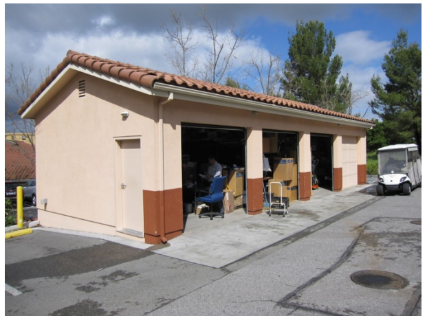
Photograph 10. Maintenance building. One of the three grease interceptors is shown at lower right.
