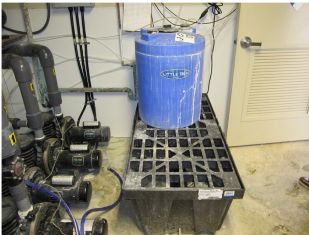
Photograph 9. Pool chemical storage.
