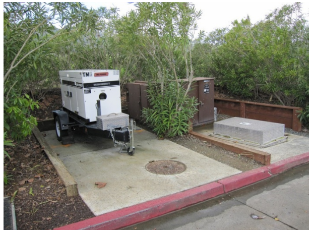
Photograph 6. Sanitary sewer lift station and generator.
