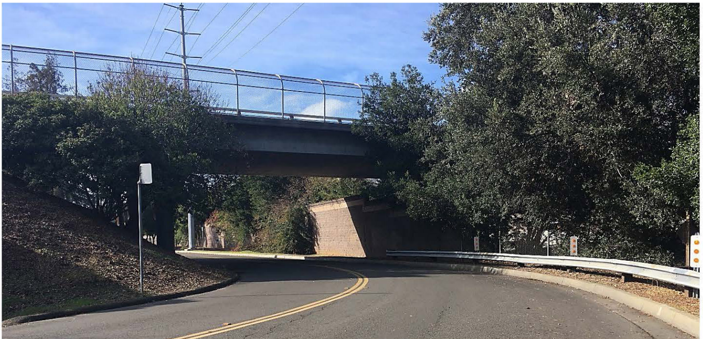
Photo 4. Viewing northwest towards the N. Blaney Avenue overpass from N. Blaney Avenue. (Central section)
